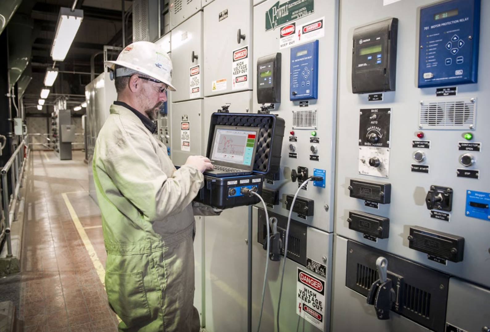
A technician using an EXP4000 analyzer connected to an EP1000 port at an MCC.
