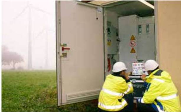
By helping detect and counteract islanding in distributed power generators, SVERKER900's ramp instrument is useful to test frequency protection.
